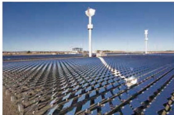
光热塔式跟踪系统 Tower Solar-Thermal System
